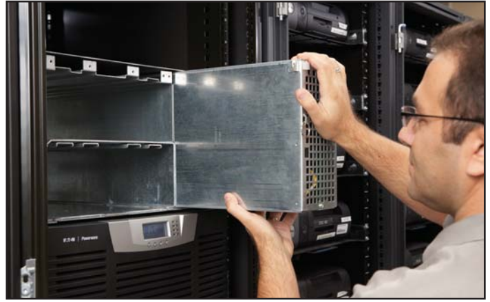
IT staff can easily install electronics modules.
