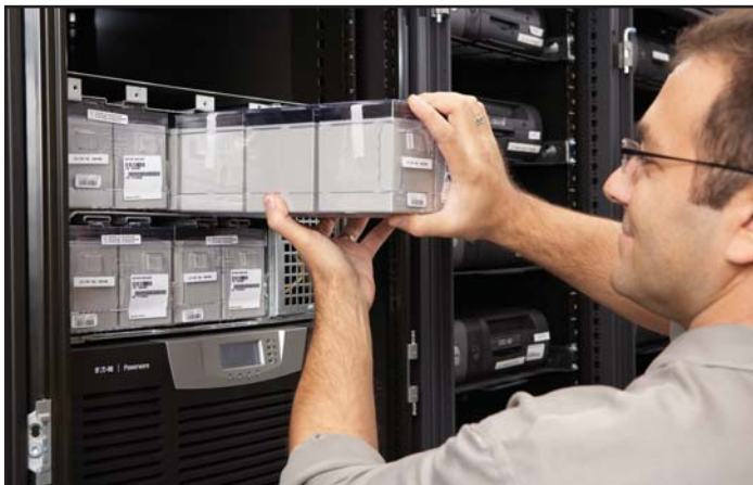
IT staff can easily replace battery modules.
