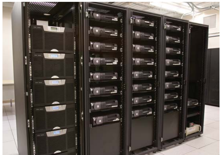
The Powerware BladeUPS remains cool even in a data center full of servers.
